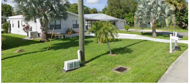
Manufactured home with elevated HVAC and drain in yard
