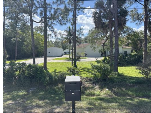
Drainage with overgrown vegetation
