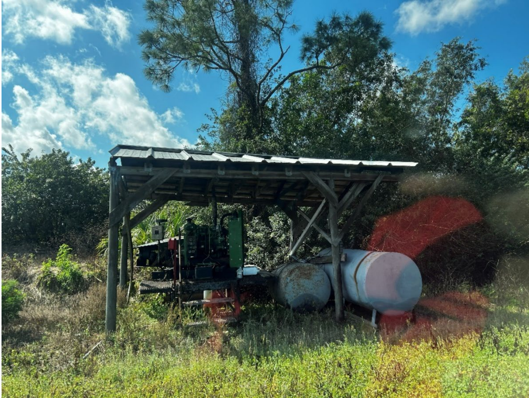
Roofed structure covering a pump station and 2 above ground fuel storage tanks
