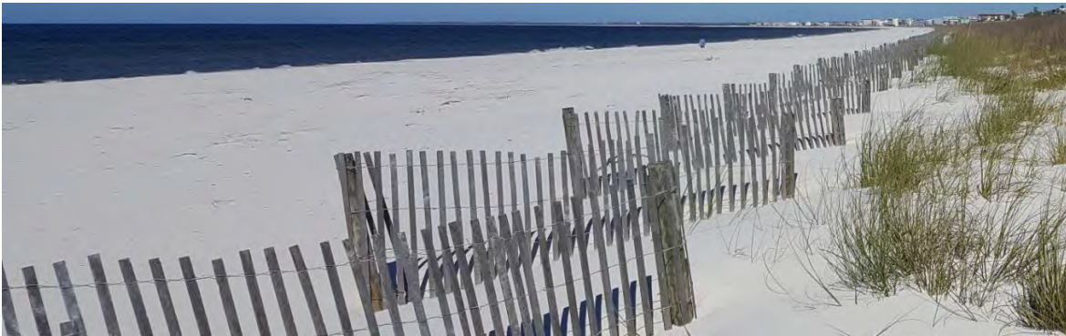
Figure 1: Sand fences installed to state of Florida specifications for the Mexico Beach dune restoration project built after Hurricane Michael. These sand collection fences have enlarged the new dune by trapping sand from the beach. Installation of sand fences in combination with planting vegetation has been a successful dune restoration method.
